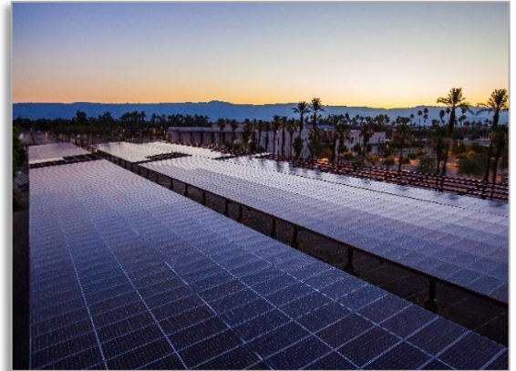
Solar Photovoltaic System
